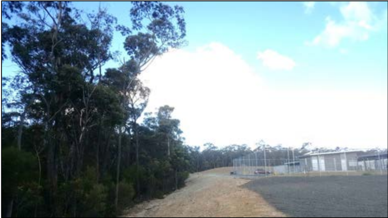
Plate 11. Looking east along the northern boundary of the 50 m gun range, construction now completed (date taken: 08/08/19).
