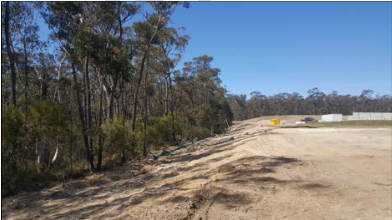
Plate 11. Looking east along the northern boundary of the 50 m gun range under construction (date taken: 29/08/18).
