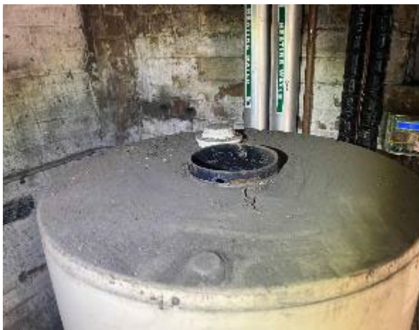
Line ID 59: Internal, Accommodation Building, Boiler House, Throughout Surfaces, Dust - Lead Detected (1,400 mg/kg)
