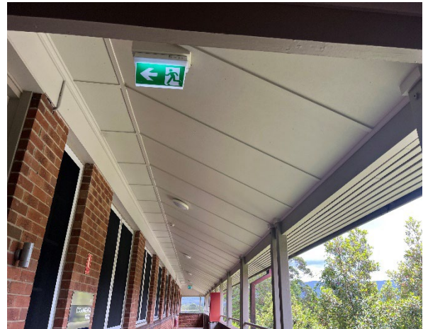
Line ID 2: External, Accommodation Building, Coolangatta, Veranda Ceiling, Fibre Cement Sheet - Chrysotile, Amosite and Crocidolite Asbestos Detected
