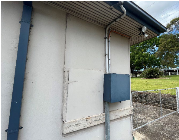
Line ID 15: External, Workshop and Silo, Maintenance Shed and Offices, South Elevation, Wall Lining, Fibre Cement Sheet - Chrysotile, Amosite and Crocidolite Asbestos Detected
