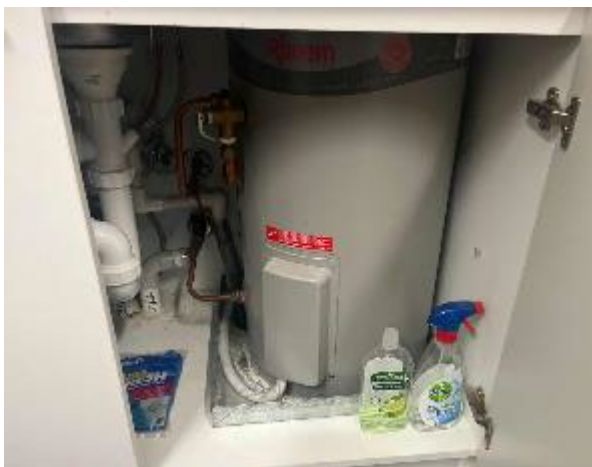
Line ID 66: Internal, Admin Building, Kitchen, Hot Water Unit, Insulation Material - Suspected SMF
