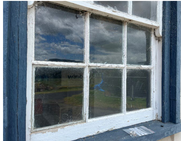
Line ID 16: External, Workshop and Silo, Maintenance Shed and Offices, Timber Windows Throughout, Window Caulking - No Asbestos Detected
