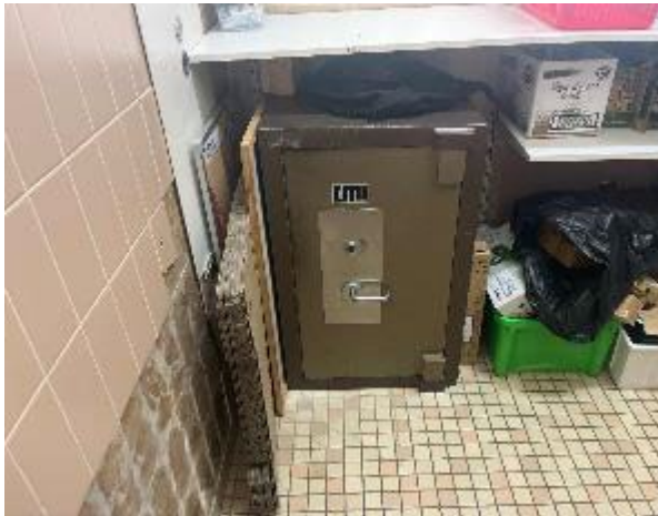
Line ID 38: Internal, Admin Building, Storeroom, CMI Safe, Internal Insulation - Suspected Asbestos
