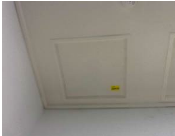
Line ID 24: Internal, Accommodation Building, GF Disabled Male Toilet, Ceiling Hatch, Fibre Cement Sheet - No Asbestos Detected
