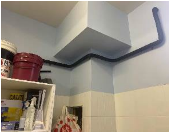
Line ID 23: Internal, Accommodation Building, GF Cleaners Room, High Level Boxing, Fibre Cement Sheet - No Asbestos Detected
