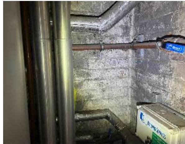
Line ID 17: Internal, Accommodation Building, Boiler House, Behind Paint to Walls, Lagging Debris - Amosite Asbestos Detected
