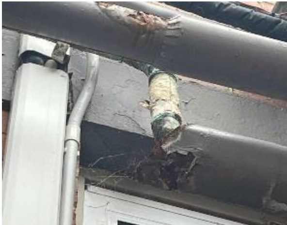
Line ID 1: External, Accommodation Building, Adjacent Boiler House, Pipes to High Level, Lagging Debris - Amosite Asbestos Detected
