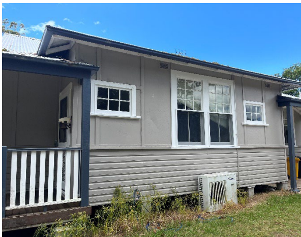
Line ID 13: External, South Residence, Verandas, Wall Cladding, Fibre Cement Sheet - Chrysotile & Amosite Asbestos Detected
