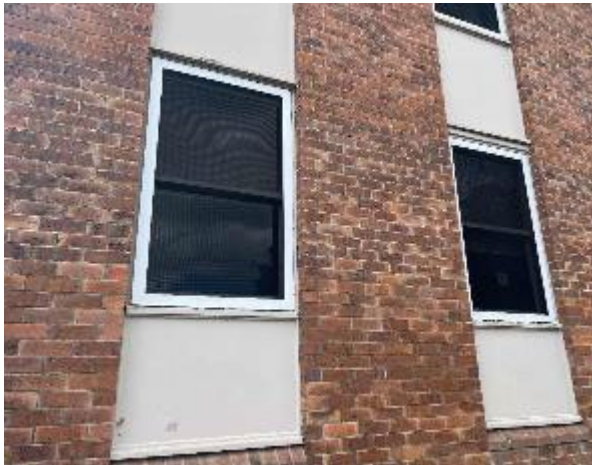
Line ID 3: External, Accommodation Building, Staff Accommodation, Above and Below Windows, Infill Panels, Fibre Cement Sheet - Chrysotile Asbestos Detected
