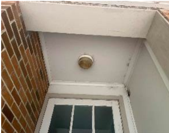
Line ID 7: External, Admin Building, Entry Area and Covered Walkways, Porch Ceiling Lining, Fibre Cement Sheet - Chrysotile, Amosite and Crocidolite Asbestos Detected
