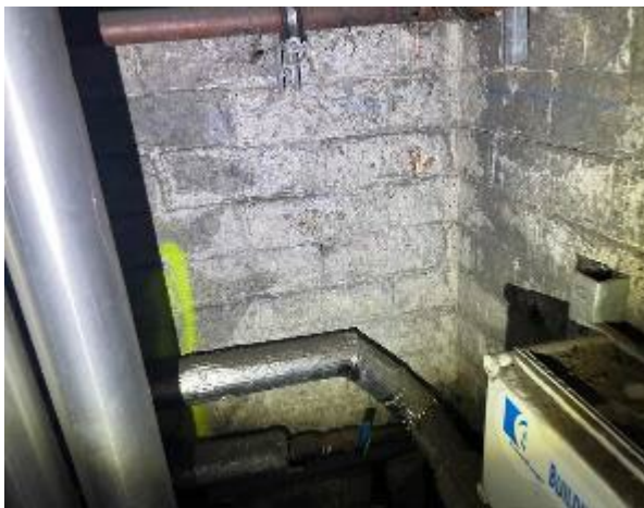
Line ID 17.1: Internal, Accommodation Building, Boiler House, Behind Paint to Walls, Lagging Debris - Amosite Asbestos Detected
