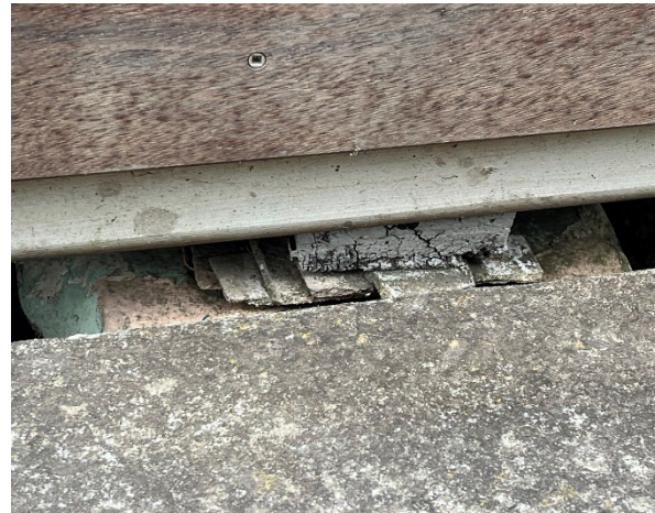
Line ID 12: External, South Residence, Verandas, Packers to Timber Deck, Fibre Cement Sheet - Chrysotile Asbestos Detected
