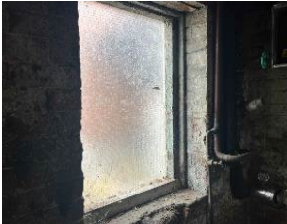
Line ID 55: Internal, Accommodation Building, Boiler House, Timber Windows, Light Blue Paint - Lead Detected (3.3% w/w)
