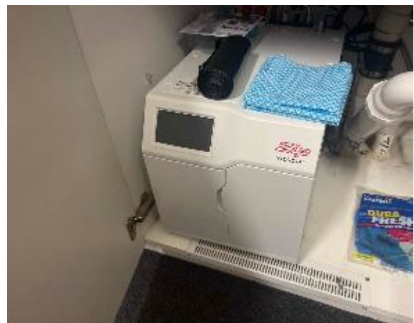
Line ID 66.1: Internal, Admin Building, Kitchen, Hot Water Unit, Insulation Material - Suspected SMF
