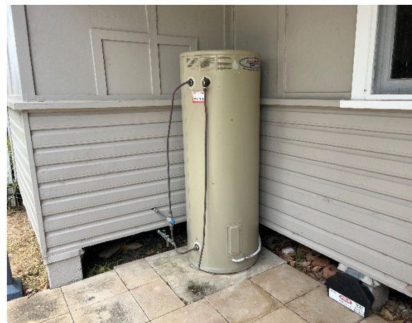
Line ID 62: External, South Residence, Verandas, Hot Water Unit, Insulation Material - Suspected SMF
