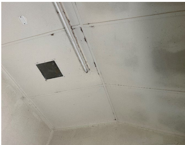
Line ID 50: Internal, Workshop and Silo, Maintenance Shed, Maintenance Building, Ceiling Lining, Fibre Cement Sheet - Chrysotile, Amosite and Crocidolite Asbestos Detected
