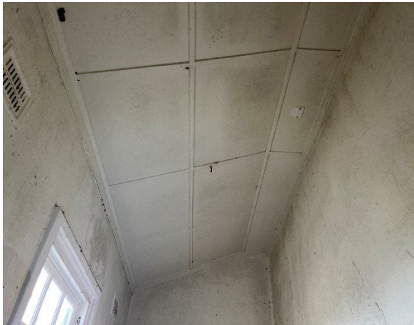
Line ID 50.2: Internal, Workshop and Silo, Maintenance Shed, Maintenance Building, Ceiling Lining, Fibre Cement Sheet - Chrysotile, Amosite and Crocidolite Asbestos Detected
