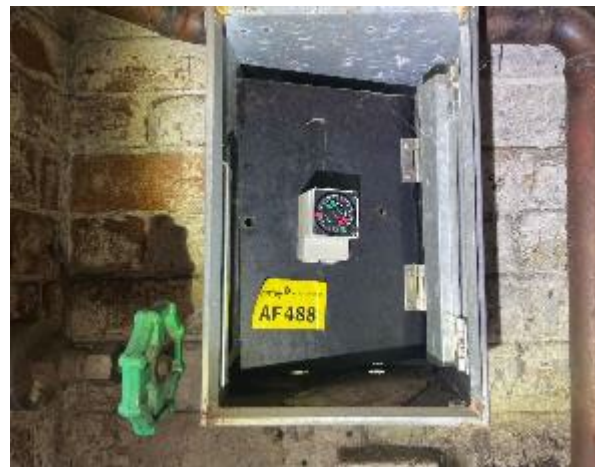
Line ID 18: Internal, Accommodation Building, Boiler House, Electrical Box Behind Water Heater, Bituminous Backing Board - Chrysotile Asbestos Detected
