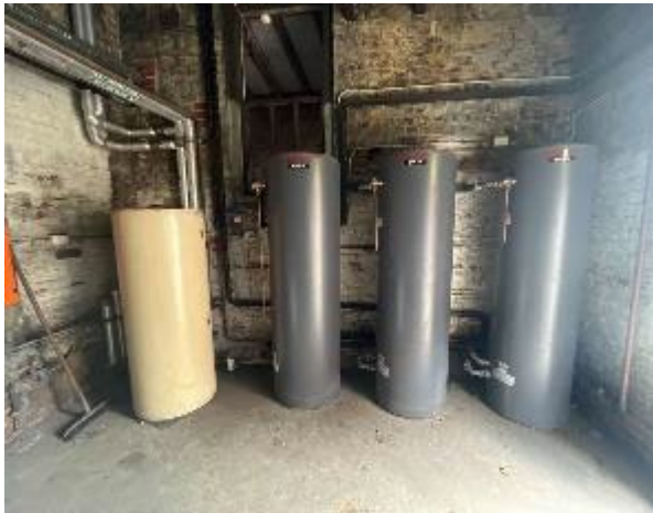
Line ID 63: Internal, Accommodation Building, Boiler House, Hot Water Units, Insulation Material - Suspected SMF
