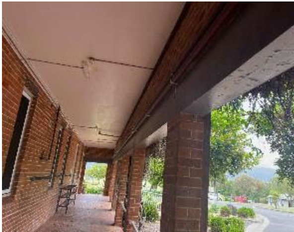
Line ID 51.1: External, Accommodation Building, Covered Walkway, High Level Bricks, Dark Blue Paint - Lead Detected (3.8% w/w)
