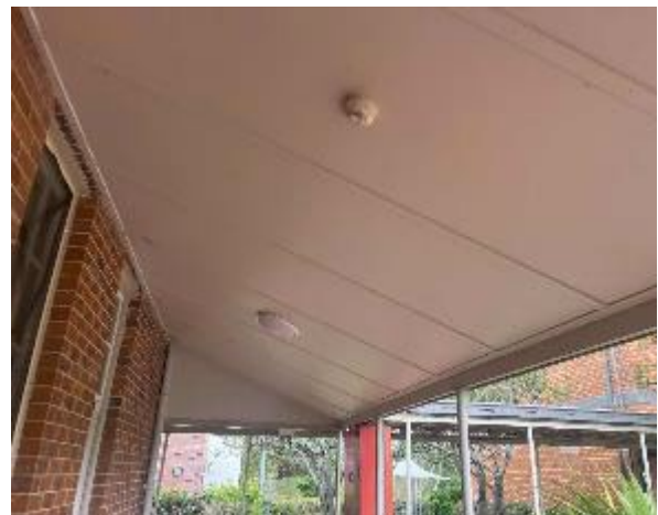
Line ID 6: External, Admin Building, Entry Area and Covered Walkways, Awning Lining, Fibre Cement Sheet - Chrysotile, Amosite and Crocidolite Asbestos Detected
