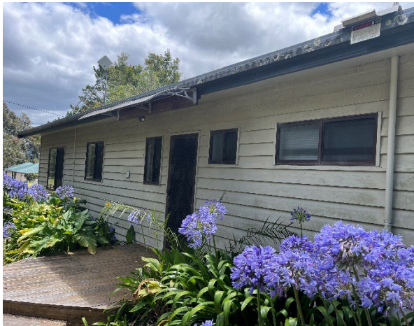
Line ID 10: External, North Residence, Verandas, Wall and Eave Linings, Fibre Cement Sheet - No Asbestos Detected
