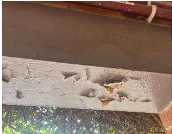
Line ID 51: External, Accommodation Building, Covered Walkway, High Level Bricks, Dark Blue Paint - Lead Detected (3.8% w/w)
