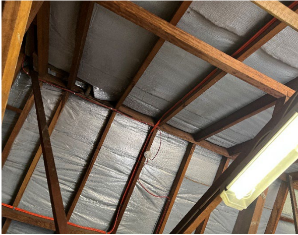
Line ID 67: Internal, Pool House, Throughout, Underside of Roof, Sarking Insulation - Suspected SMF
