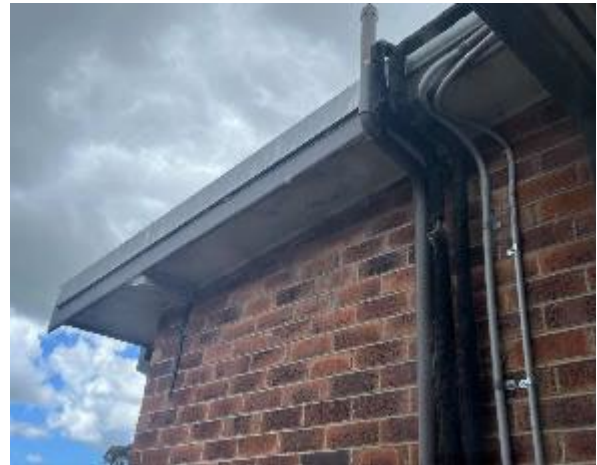
Line ID 4: External, Accommodation Building, Staff Accommodation, Eave Lining, Fibre Cement Sheet - Suspected Asbestos
