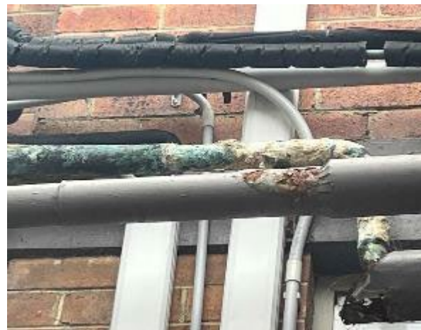
Line ID 60: External, Accommodation Building, Adjacent Boiler House, Pipe Insulation, Insulation Material - Suspected SMF
