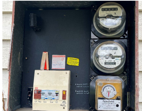
Line ID 9: External, North Residence, Verandas, Side of House, Fuse Box, Electrical Backing Board - Suspected Asbestos
