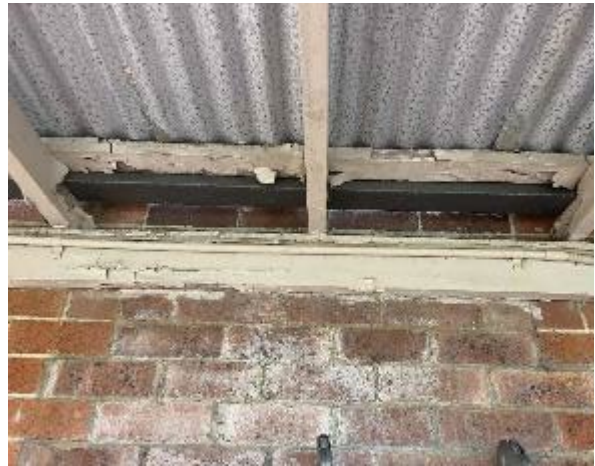
Line ID 52: External, Accommodation Building, Covered Walkway, Timber Work of Metal Roof Section, Beige Paint - Lead Detected (0.26% w/w)
