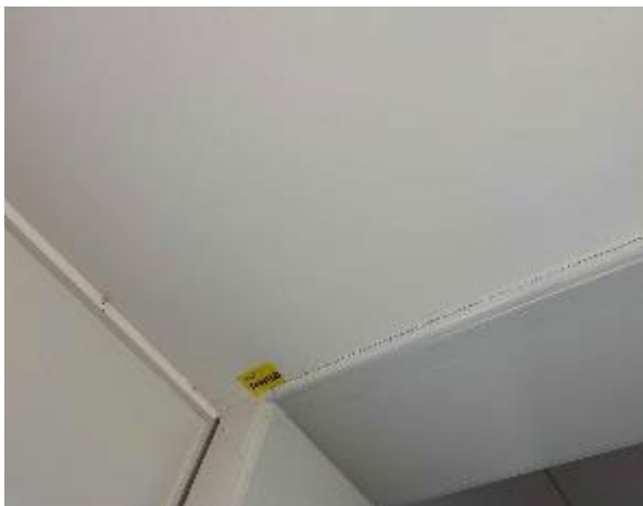
Line ID 30: Internal, Accommodation Building, L1 Corridor to Staff Accommodation, Ceiling Lining, Compressed Cement Sheet - No Asbestos Detected
