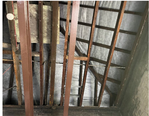
Line ID 65: Internal, Accommodation Building, Boiler House, Underside of Roof, Sarking Insulation - Suspected SMF
