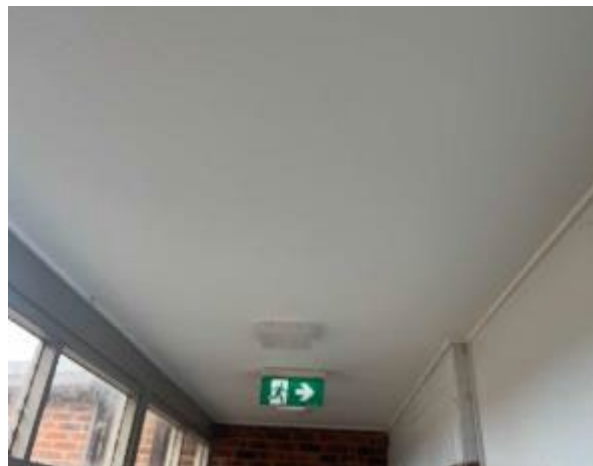
Line ID 30.1: Internal, Accommodation Building, L1 Corridor to Staff Accommodation, Ceiling Lining, Compressed Cement Sheet - No Asbestos Detected
