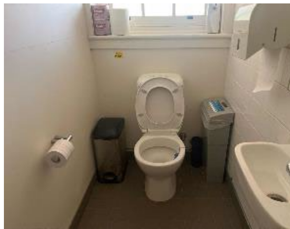
Line ID 37: Internal, Admin Building, Ladies Toilet, Wall Lining, Fibre Cement Sheet - No Asbestos Detected
