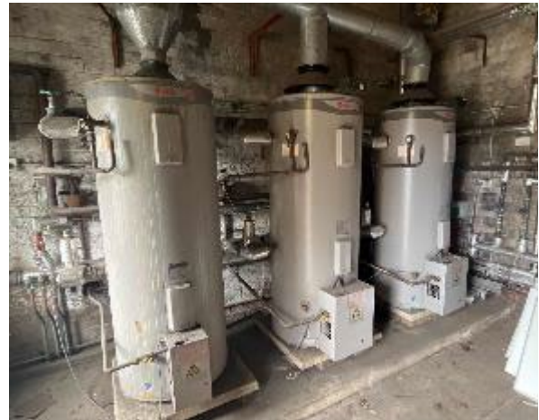
Line ID 63.1: Internal, Accommodation Building, Boiler House, Hot Water Units, Insulation Material - Suspected SMF
