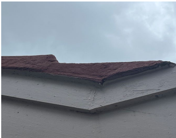
Line ID 42: Internal, Pool House, Throughout, Verge Lining to Roof Tiles, Fibre Cement Sheet - No Asbestos Detected
