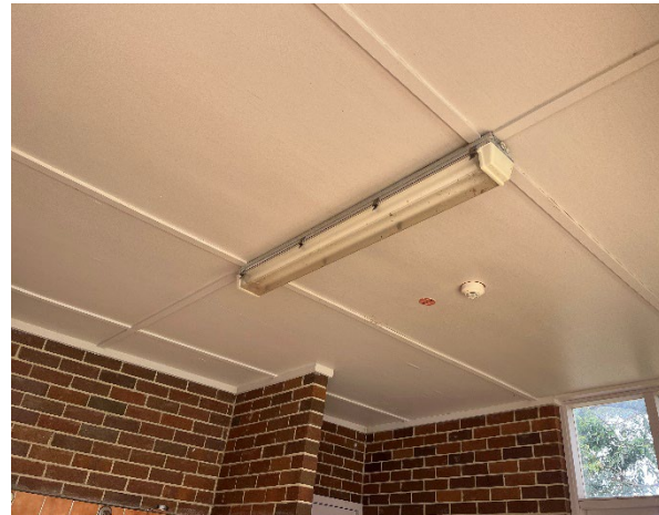
Line ID 41: Internal, Pool House, Throughout, Shower Area, Ceiling, Fibre Cement Sheet - No Asbestos Detected
