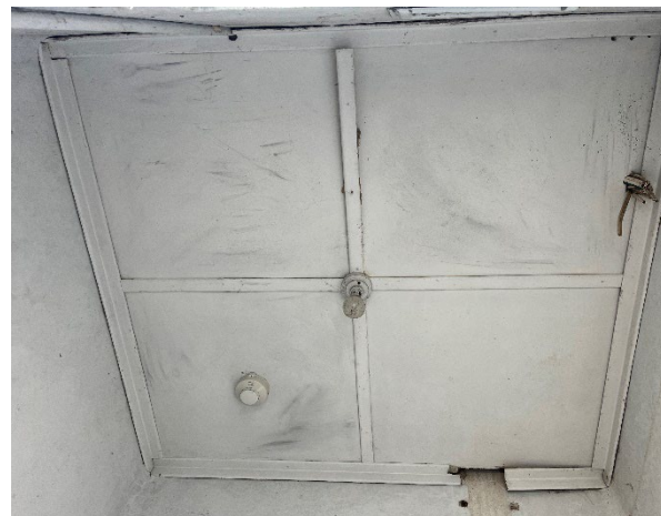
Line ID 50.1: Internal, Workshop and Silo, Maintenance Shed, Maintenance Building, Ceiling Lining, Fibre Cement Sheet - Chrysotile, Amosite and Crocidolite Asbestos Detected
