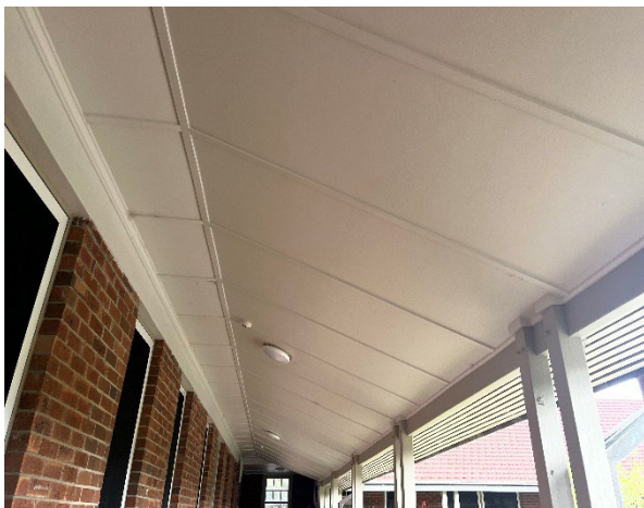
Line ID 5: External, Accommodation Building, Watson & Shoalhaven, Veranda Ceiling, Fibre Cement Sheet - Chrysotile, Amosite and Crocidolite Asbestos Detected
